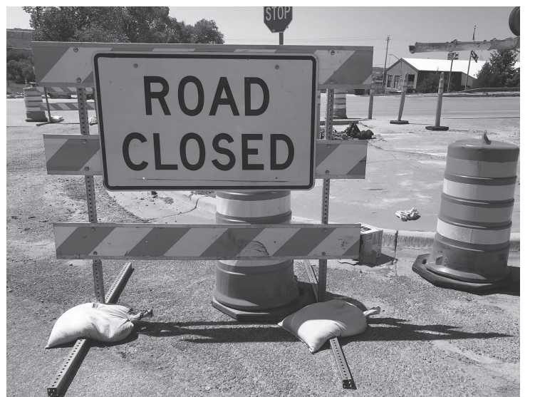
Road closed signs have made many appearances in Newcastle throughout the summer. Wyoming Department of Transportation engineer John Leahy, however, said residents need only worry about construction for about two more months, as it will be wrapping up mid-September. (Photos by Abby Gray)
