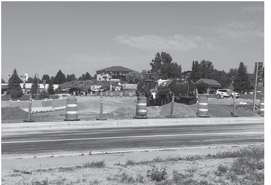
Some of the construction at the four-way intersection in Newcastle was done to give cars a lane to travel rather than a long detour around town. All cones will be pulled back off the road beginning July 27, to prepare for the traffic through down during the Sturgis Motorcycle Rally.
